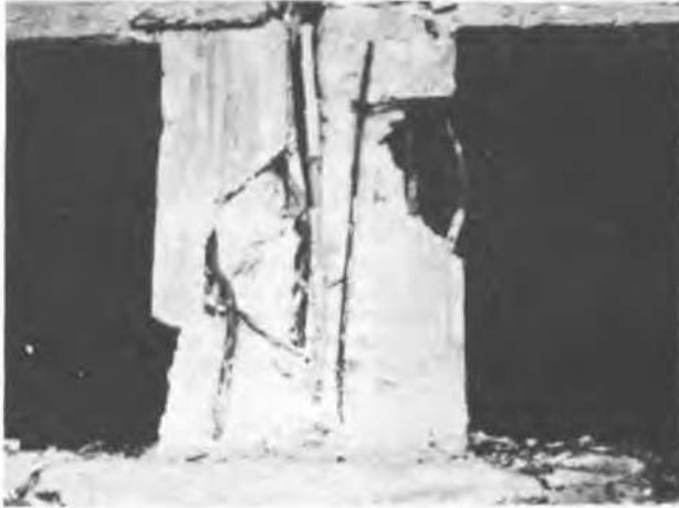
Fig. 1 Column Destruction at Expansion Joint (Site A)
