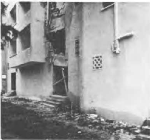
Fig. 8 Building at Site C, Showing Settlement of 30 cm in Right Hand Portion of Building
