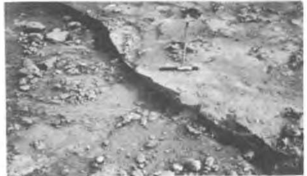
Fig. 9 Photograph of expansion crack of Fig. 8
