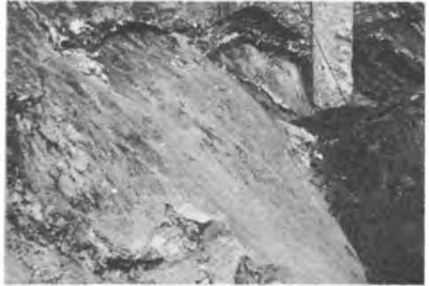
Fig. 11 Slickensided surface that caused a localized sliding of soil between soldier piles 10 ft or 3 m apart in an excavation 60 ft or 18 m deep. Width of photograph approximately 10 ft or 3 m
