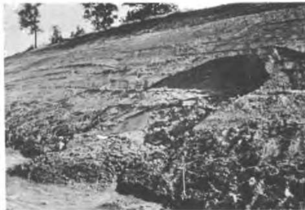
Fig. 10 Local slide in a railroad cut 75 ft or 22 m deep in weathered diorite in North Carolina which commenced on two intersecting slickensides similar to Fig. 5
