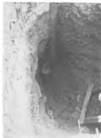
Fig.10 Photograph of the displaced plastic tube and destroyed concrete filling of the observation boring No.11.
