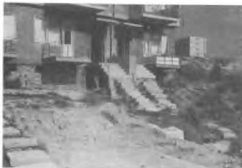
Fig.8 Depression of the ground in front of the house (H) at the edge of the sliding mass along the X-X axis.
