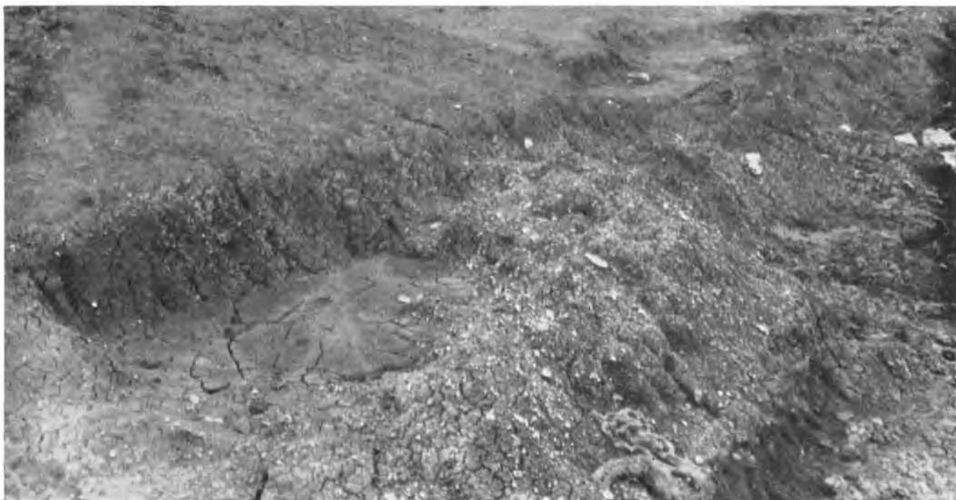
FIG. 4. Instability of the base of fill already built to partial height without treatment.
