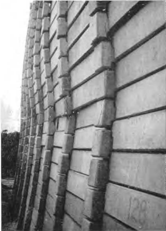
FIG. 3. Outward bulge of upper part of crib wall.
