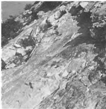
FIG. 3. Gliding deconsolidation fissure in flinty chalk.
