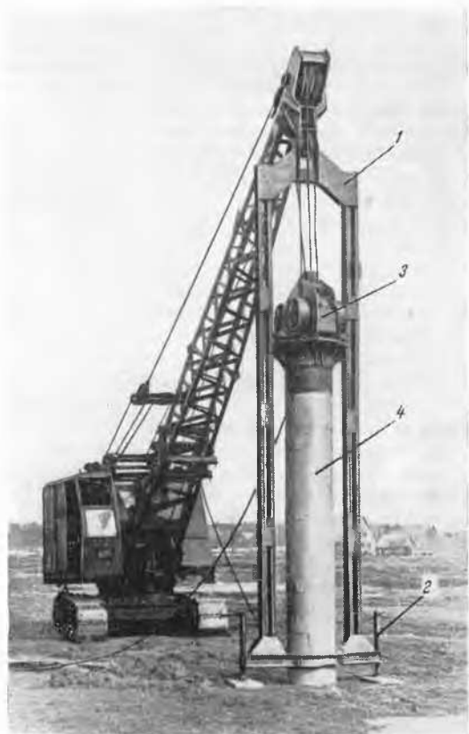
Fig. 3 The vibro-grab unit for excavating trenches (designed by A. S. Golovachjoff, V. I. Chernjajeva and others).
