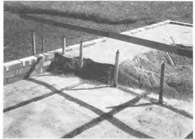
Fig. 5 Protected Area under Construction Showing Bituminous Felt Coarse Sand, Brick Wall, Concentric Shrinkage Gauges and Reference Beam Aire de protection en construction
