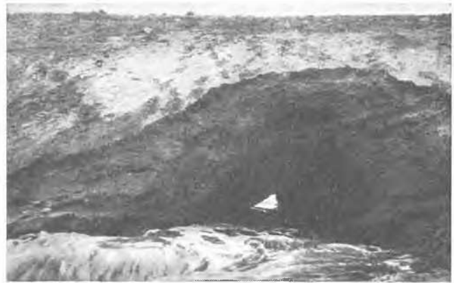
Fig. 1 View of Failure of Dam, Case B Vue de la rupture de la digue B
