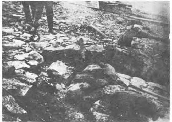
Muirhead reservoir. Arched deformation of stone pitching
