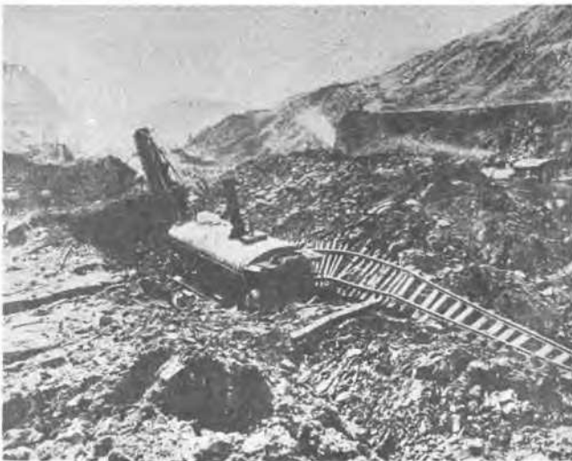
East Culebra slide showing upheaved material between stations 1746 and 1758. Looking south, Febr. 6, 1913.
