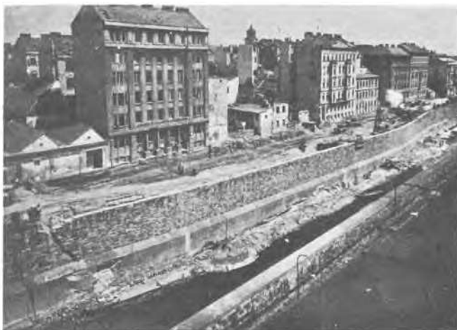
Outside front view of the displaced shore wall, taken downstream from a roof at right shore on 27th May 1946.
