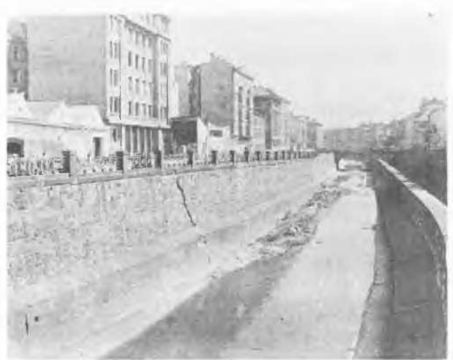
Downstream view of "Wienfluss"-creek, taken from "Wackenroderbrücke" in April 1946, immediately after displacement of left shore wall.
