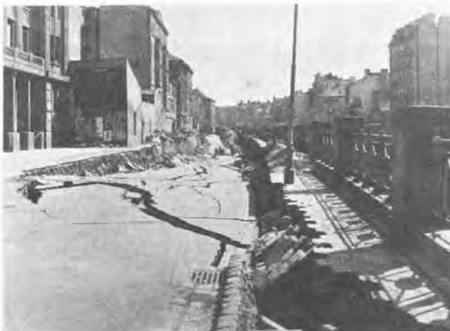
Downsettled "Linke Wientelle"-street on back of displaced creek wall. View downstream, taken in April 1946 immediately after wall displacement.
