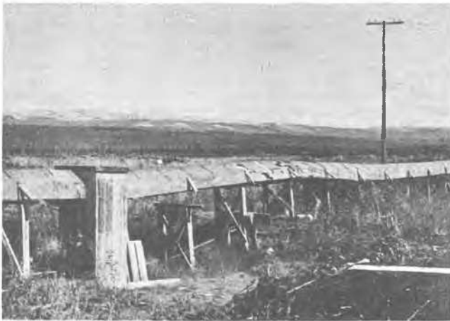
A cumulative heave of twenty inches, of a cover box for service lines is shown here. One trestle in the foreground was anchored in permafrost so that it did not move.
