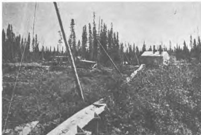
The pole line here was heaved out of the ground by frost action. Similar heave is indicated in the short post under the box for service lines along the pole line.
