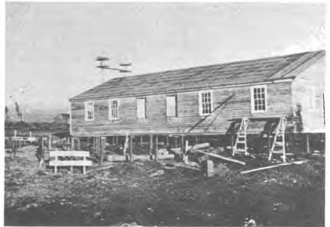
A light frame building set on steel piles. More piles are shown in the foreground.
