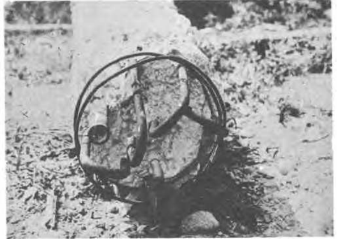
Base of the extracted pile No. 11. Note on the left the grouting pipe.
