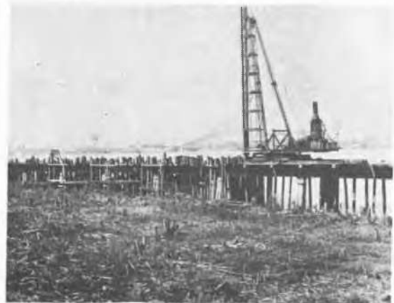
Pile driving rig No. 1 Vulcan 5,000-pound single-acting steam hammer on top of old steel girder frame.
