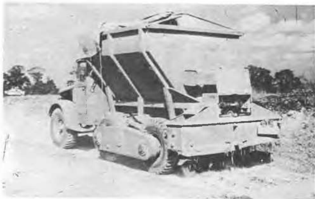
Lime - spreading lorry spreading 4 tons of cement using one main longitudinal worm and two co-axial transverse worms.
