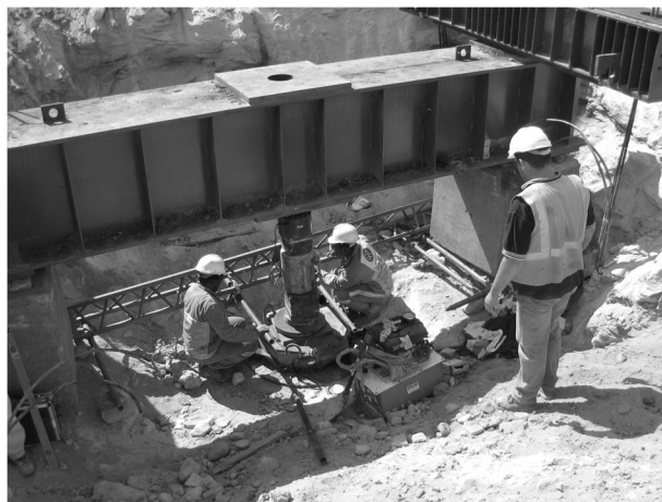
Figure 2. LPLT arrangement at final depth, Test B, showing reaction beam, load cell, hydraulic jack, plate and reference beam.
