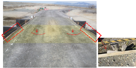
Photo 1. Condition of the surface of the road section on the embankment.
