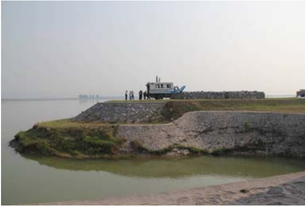
Figure 3. Assessment location alongside the Yellow River during the installation of the sensors.
