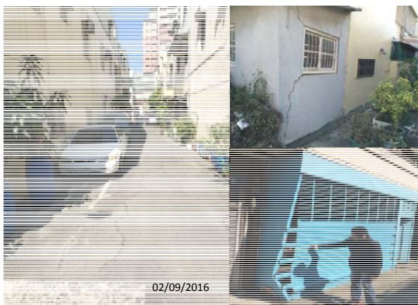
Figure 6. The settlement on the road and shallow founded houses settled on at Locality 4 and 5. Some damages were found on the extended structure and mostly the main structure remains fine
