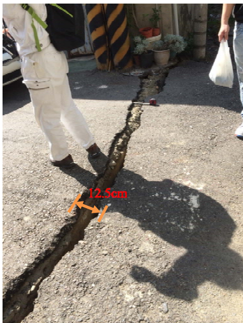
Figure 3(b). Lateral spread at Locality 1. The 12.5cm gap at the top of the slopped road.
