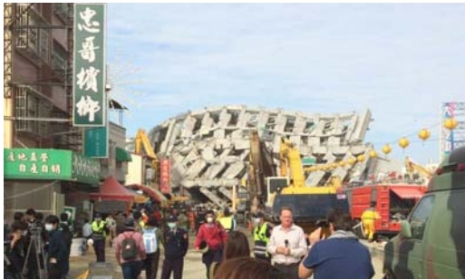
Figure 1. The severest damaged spot in 2016 Meinong earthquake. 116 deaths are reported in this collapsed 16th floor building due to structure damage.
