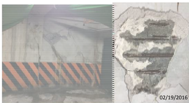
Figure 7 the damages of the walls and columns of basement of a relative tall building (Building C) in Shi- Din area. The rusted steels were found inside the cracks of the wall.
