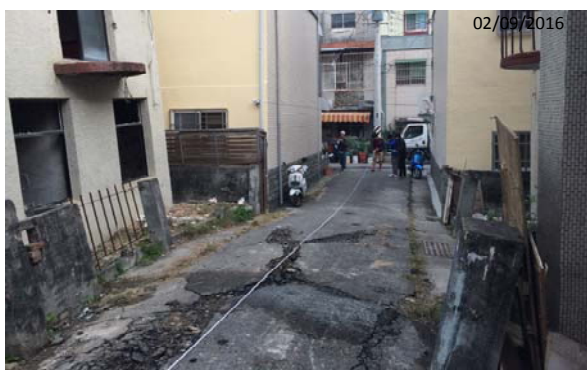
Figure 3(a). Lateral spread at Locality 1. The heave at the middle of the road is as much as 5-7 cm.
