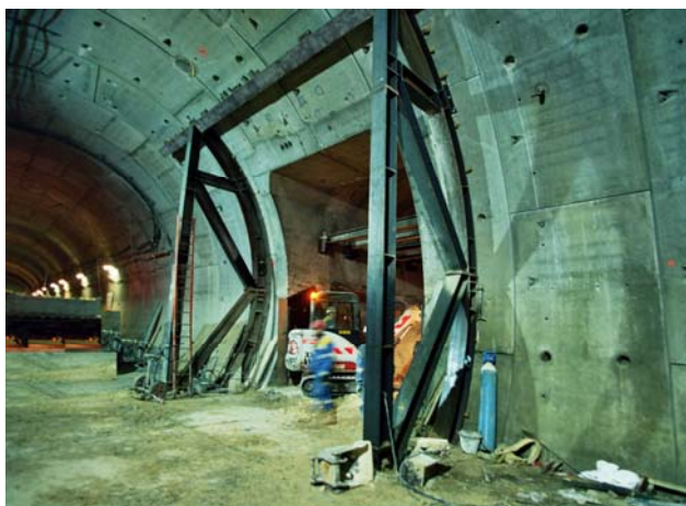
Figure 4. 'Half-moon' support frame in A86 Sotatop Tunnel in France.
