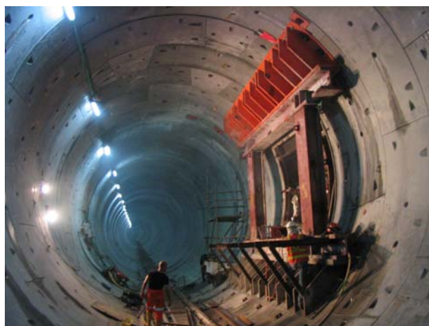
Figure 3. Steel lintel and sill beams in conjunction with steel props in Kowloon Southern Link Tunnel in Hong Kong.
