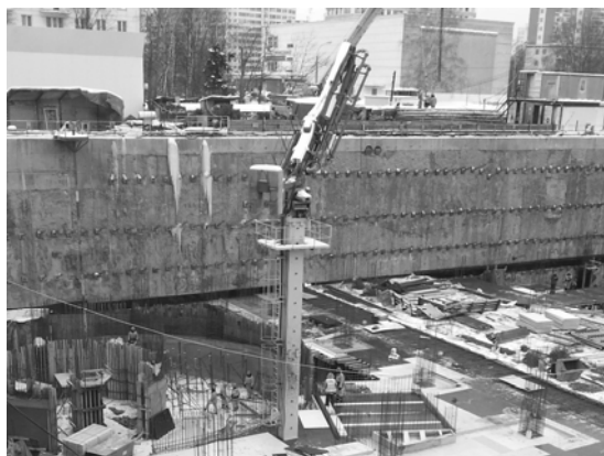
Figure 2. SBMA anchors with additional grouting; a — scheme of anchor; b — photo of the site
