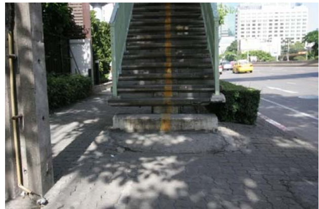
Figure 2. Pavement settled away from piled footbridge as a result of surface settlement
