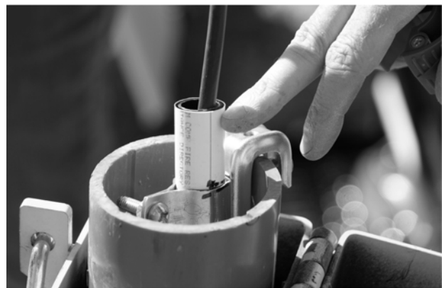
Figure 6. Special installation fixture used to lock SAAV in position. Note the PEX tubing at the top of the SAAV has been cut back so that the lid for the casing protection can be closed.
