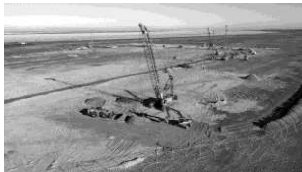
Figure 3. Job site picture. Cable cranes on the site in Cuxhaven in front of the Elb.
