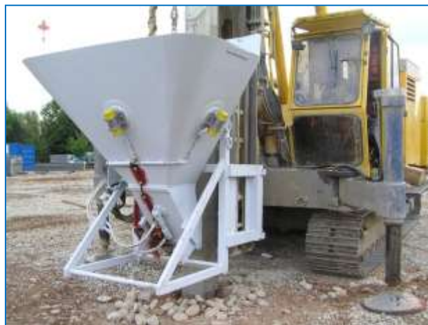
Figure 3. New sand hopper for the vibrocat
