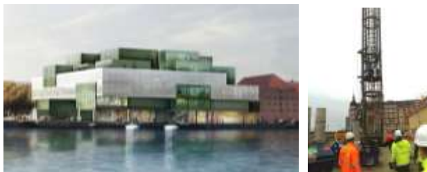
Figure 1. (a) Project BLOX, Copenhagen harbour; (b) Lowering of reinforcement cage with O-cell into temporary casing.
