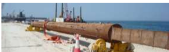
Figure 9. (a) Principle of O-cell testing; (b) test pile with reaction pile protruding (note shear keys on both piles).
