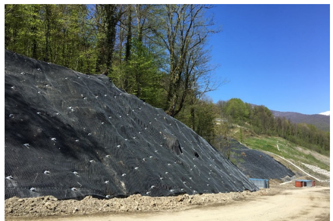
Figure 3. Slope stabilization by Ischebeck TITAN soil nails combined with a Geobrugg TECCO steel mesh, Alpika Service, Sochi, Russia
