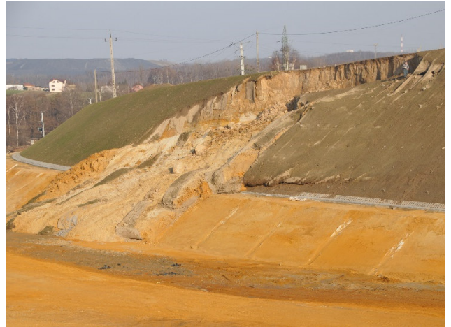
Figure 2. Slope failure, highway A1 in Poland.
