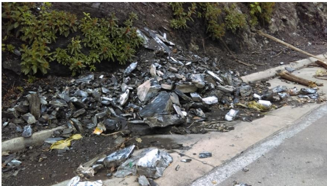
Figure 6. Rock Blocks fall to the road.
