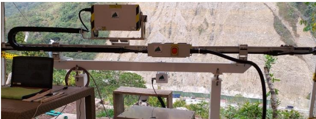
Figure 8. LISA type radar installed for 24/7 slope monitoring.
