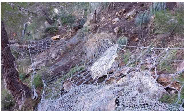
Figure 2. Pictures of Formentor rockfall event with severely damaged lying dynamic barrier and stopped rock blocks close to the Ma-2210 road.
