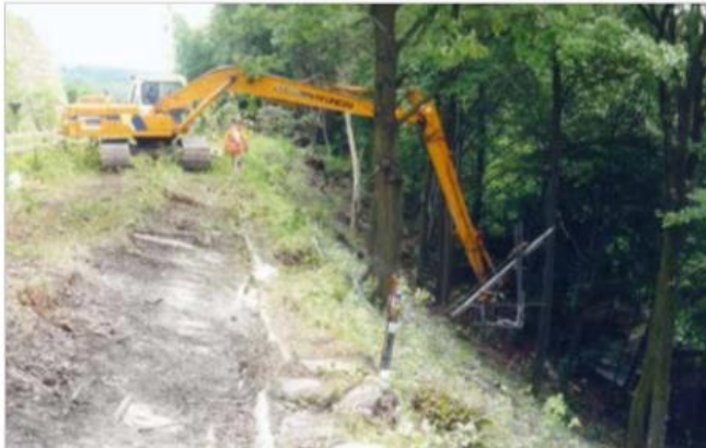
Figure 7: An example of soil nail installation in a forested area (Friedrich Ischebeck GmbH 2019).
