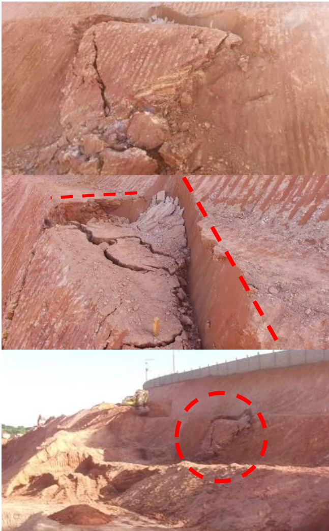
Figure 4: Front, top and side view of the failure (Sérgio Velloso Projetos collection)
