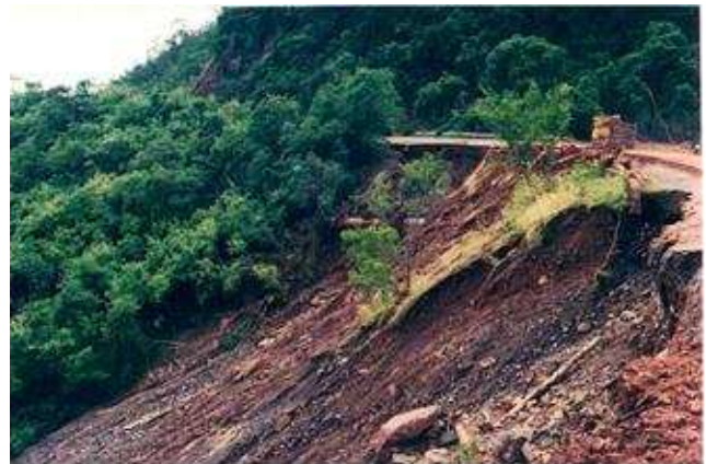
Figure 2. View of the embankment's body erosion caused by a debris flow.
