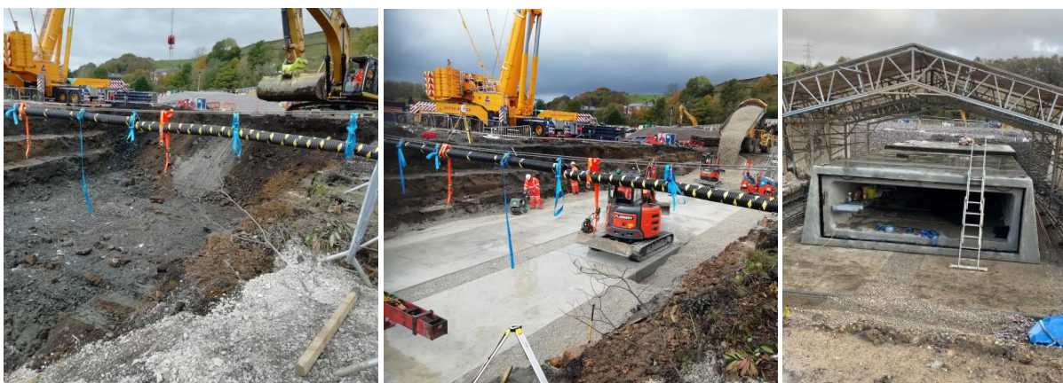
Figure 7: Photos of the construction works from left to right: (a) excavation in dry ground, (b) laying the foundation, and (c) the box culvert after the reinstatement of the railway line.
