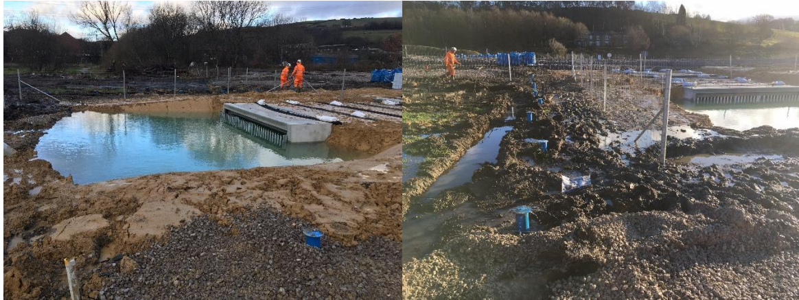
Figure 8: Photos of the box culvert after the dewatering system was turned off, from left to right: (a) Gale East (b) Gale West .
