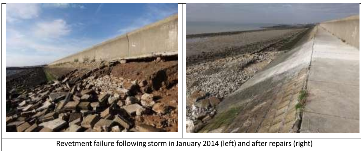
Figure 4: Chapman Sands revetment failure (Courtesy: Environment Agency).
