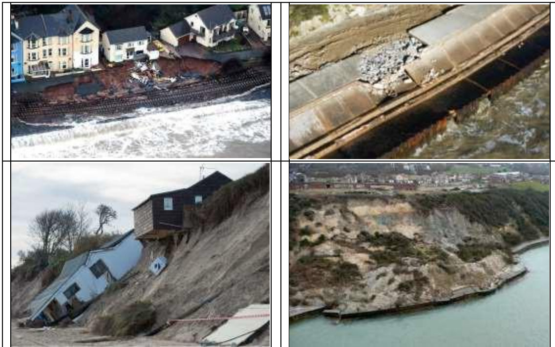
Figure 1: Examples of the impacts of coastal storms and vulnerability of infrastructure; Top left: Dawlish, Devon, 7th February 2014; Top right: Ventnor, Isle of Wight, 3 rd November 2022; Lower left: Hemsby, Norfolk, 6th December 2013; Lower right: Totland Bay, Isle of Wight, 26th December 2012. Images courtesy: Network Rail, Alamy Stock Photo, Solent Coastguard.
