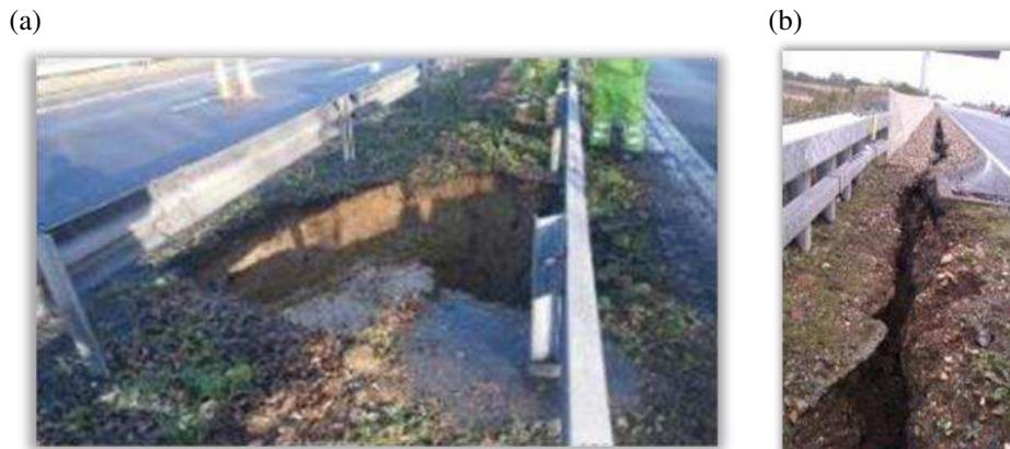
Figure 1: (a) In February 2014, heavy rainfall led to the formation of a cavity in soluble ground, which led to the total closure of the M2 between Junctions 5 and 6; (b) Tension cracks as a result of shrink-swell of susceptible embankments on M11 between Junction 5 and 6. This resulted in closure of hard shoulder and multiple geotechnical interventions (Source: National Highways).
