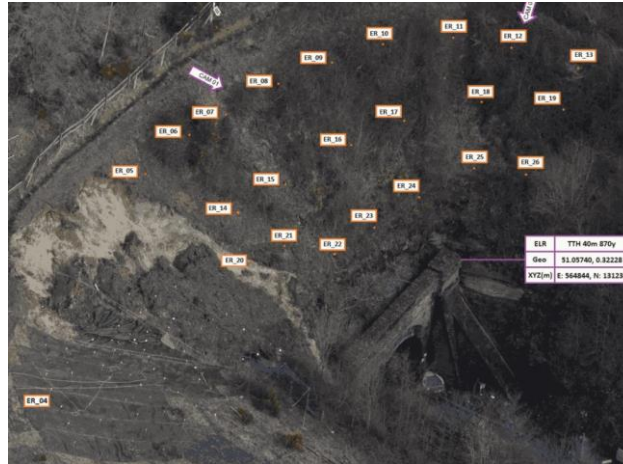
Figure 8. Aerial view of slope failure above Wadhurst Tunnel
