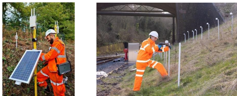
Figure 4. Left - installing Edgehub Gateway, 4G camera and solar panel. The Edgehub collates sensor and image data and transfers to stakeholders via the cellular network. Right - installing tilt nodes on metal stakes.
