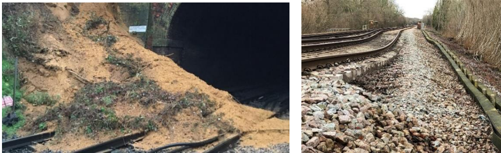
Figure 3. Steep cutting slopes are prone to landslide after heavy rain (left) and track damage can be caused by flooding and damage to supporting materials (right)
