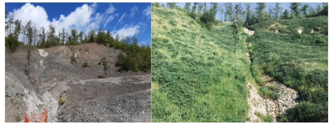
Figure 8. Hydraulic regulation works implemented directly on the natural soil on the slope following the collapse of the channels built with cemented stone blocks (Autostrade per l'Italia site on the A1 motorway - Bologna)
