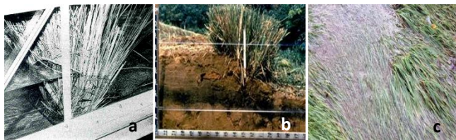
Figure 8. a) and b): hydraulic jumps in the intake works, constructed in situ on the existing substrate with emergent plants, to reduce water velocity; c): protective lining with prostrate deep-rooted species to prevent erosion of the bed and side-walls
