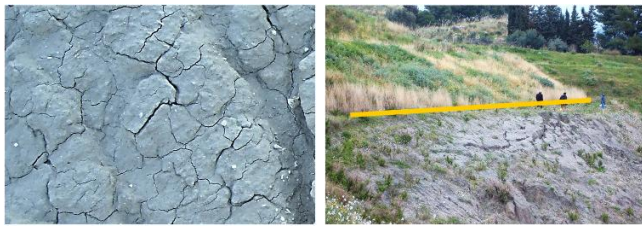
Figure 5. Menfi (AG) quarry: clay cracking and consequent hydrogeological instability; above the yellow line, the anti-erosion intervention that limited the soil cracking
