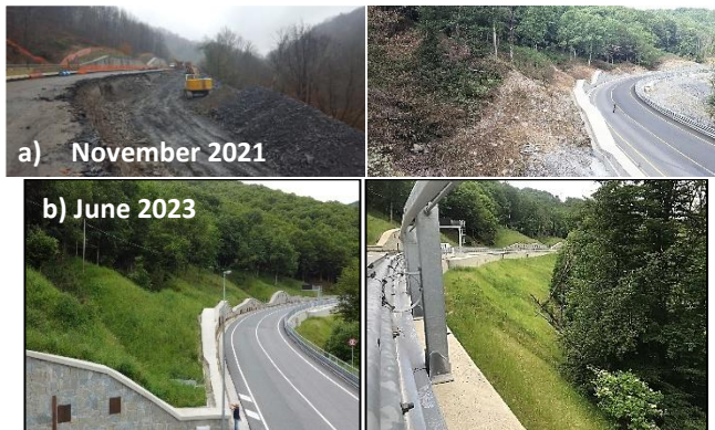
Figure 3. Torriglia (GE) – ANAS Construction Site; a) unsuccessful erosion control and hydraulic regulation implemented directly on unprocessed material; b) after the Prati Armati application: no erosion-related issues observed and surface water management installed on the untreated soil
