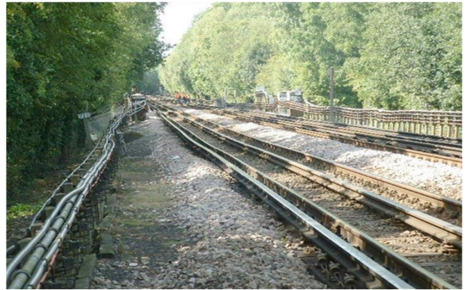
Figure 1. Typical photo showing presence of mature vegetation and seasonal deformation of track and lineside services
