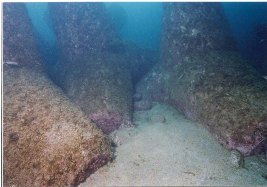
Fig. 2 - Video-captured scour hole
