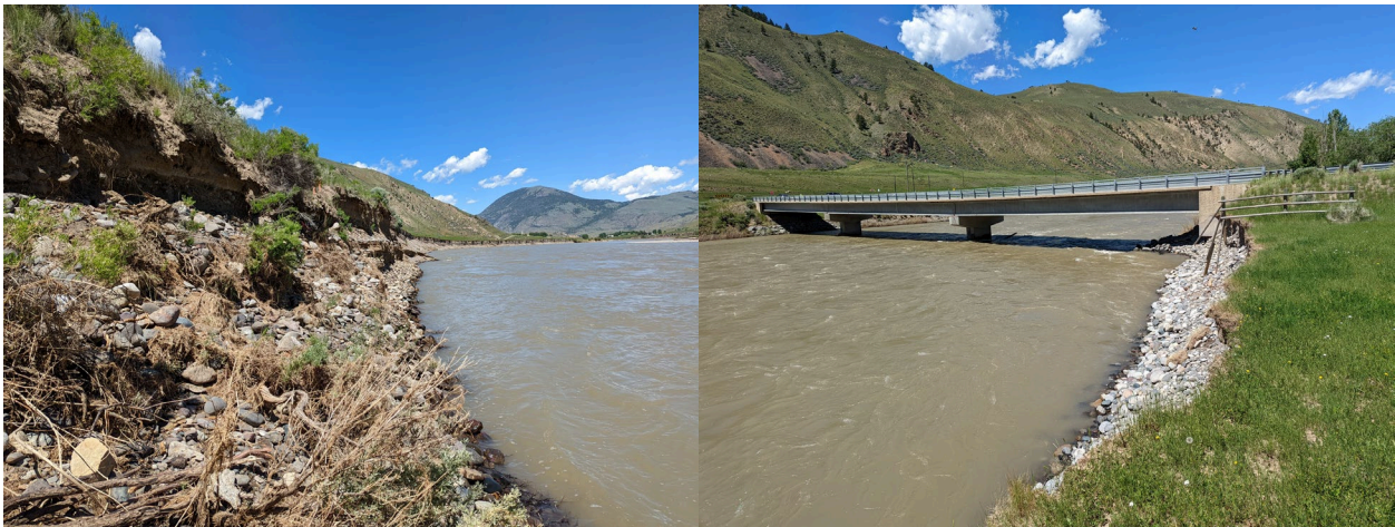
Figure 6. Erosion at the southwestern riverbank downstream of the bridge.
