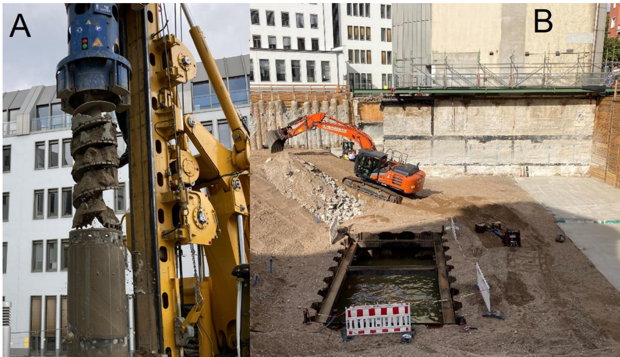
Figures 4. CFA piles during the excavation (A). pit excavation within excavation (B)
