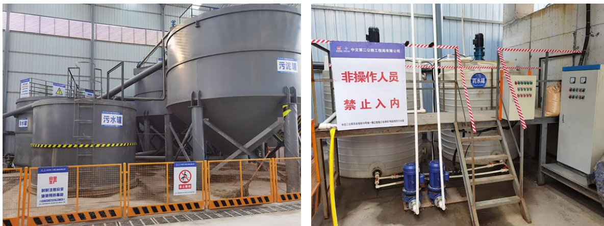
Figure 7. Slurry tank, clean water tank and flocculation tank (left). Medicine tank (right)
