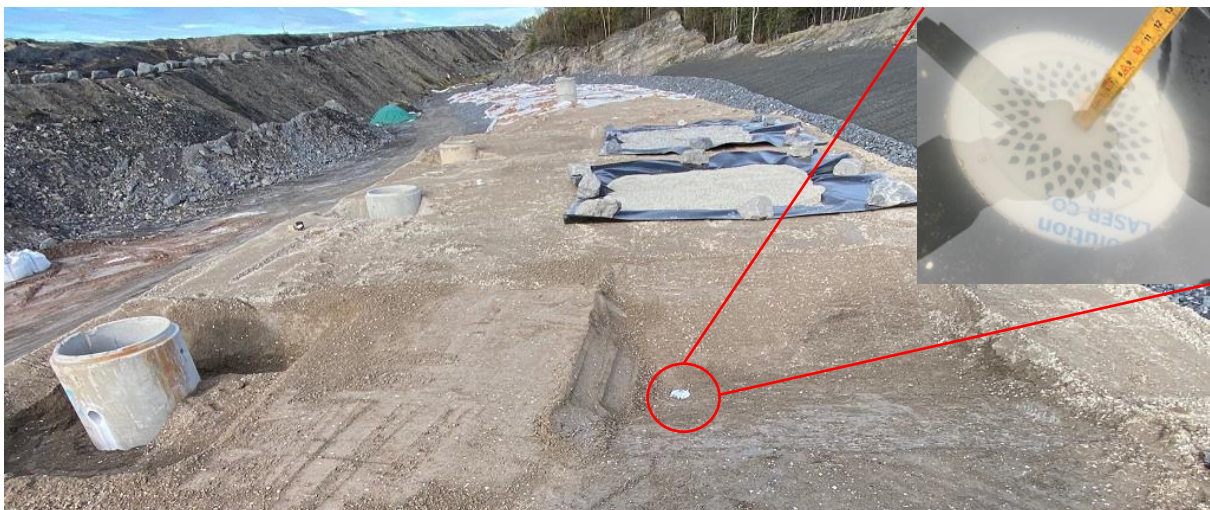
Figure 2. Construction of lysimeters. The embedded picture shows the drain during a percolation test after the geomembrane was laid out.
