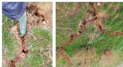
Figure 4. Drying cracks (left in the plateau area upstream of the site)
