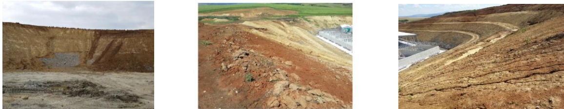
Figure 1. Local instability phenomena and (at right) initial remediation (berms)
