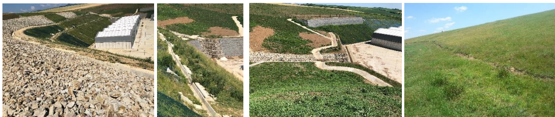
Figure 2. Final works, including drainage, mechanical consolidation works, hydrological measures; at right signs of ongoing instability
