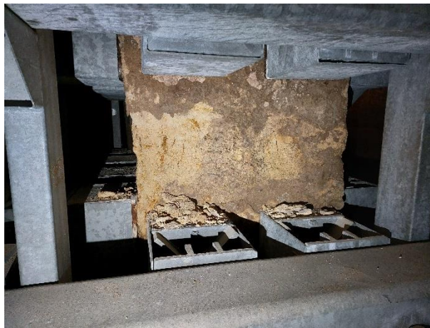
Figure 8. Pillars alteration at the base, between the metal frames (Carpentier, 2024)
