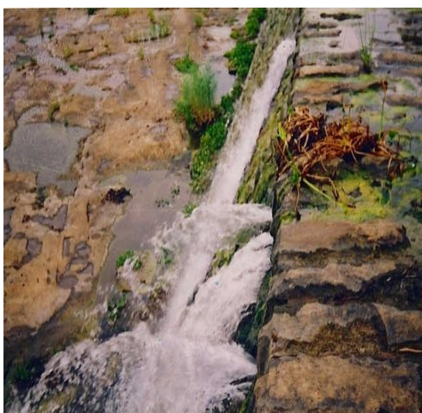
Fig. 3 Leakage through the Dam before treatment
