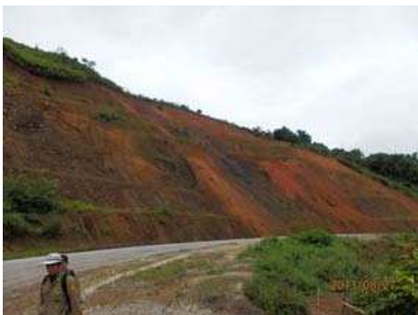
Fig 1. A typical slope failure in the road network.
