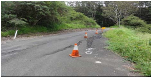
Fig. 2 Landslide re-activated by 2013 rain event
