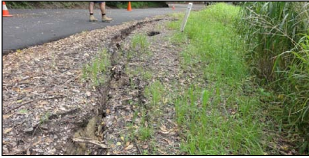
Fig. 1 Site failure by 2010-2011 rain event
